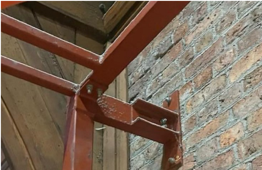
P06a Steel wall bracket and supporting frame fixed directly into historic brick masonry beside a timber opening. Remove the bolts without twisting or levering the bracket against the brick face.
